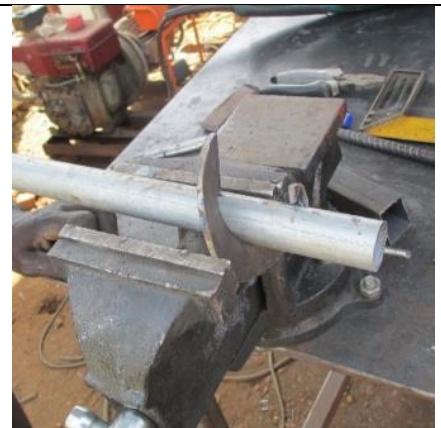
Photo 15. You can also bend the plate by welding it on the pipe and hammer it. Here the pipe is 3/4" GI
