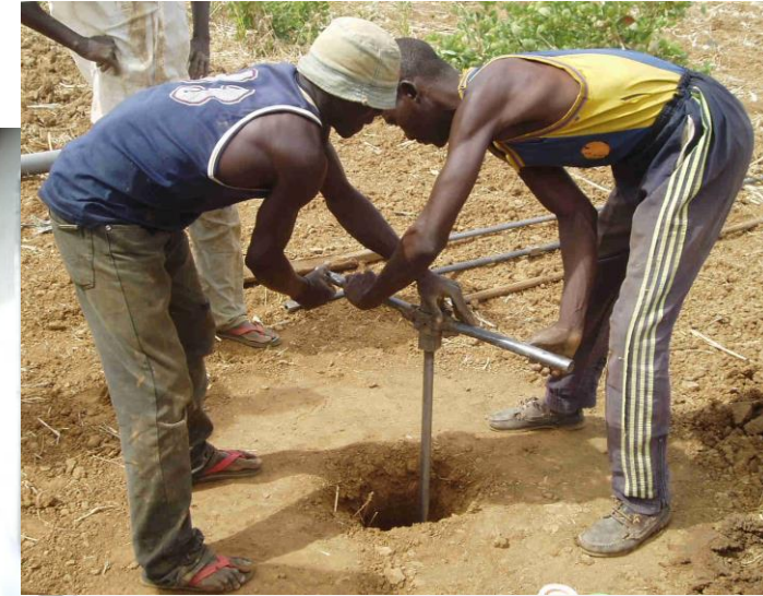
Different manual drilling techniques in use in urban Nigeria and rural Niger (Photos: Kerstin Danert)
