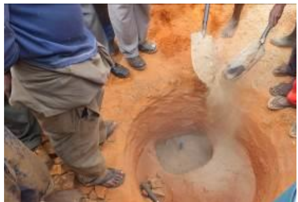
After the PVC pipe is placed, the hole is filled. If gravel is used fill up until 1 meter from the top and fill rest with sand. As used for construction.
