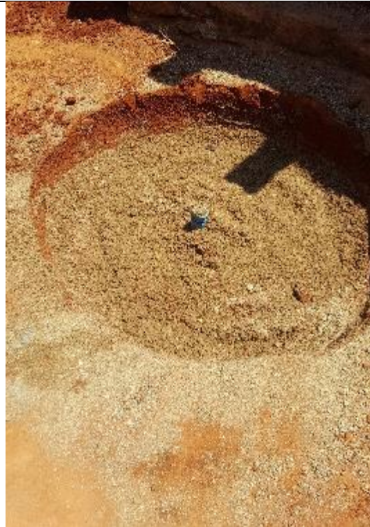
The hole is filled, if available use small gravel. If not available use sand. Make sure the PVC pipe is covered.
