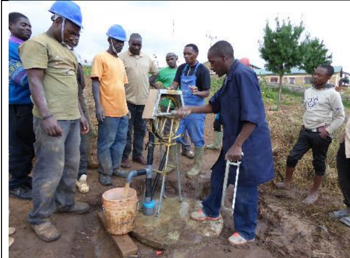
Photo 31 . Developing the well. Here a Rope pump model 2 mounted on a prefabricated well cover
