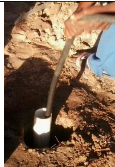
Photo 27. Push the bag down gently with the poly pipe. Avoid bag damage! Leave 2 days to cure before starting to pump
