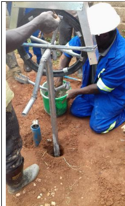
Photo 28 Developing the well. Here a Rope pump model 4 (one leg) installed 15 cm besides the well
