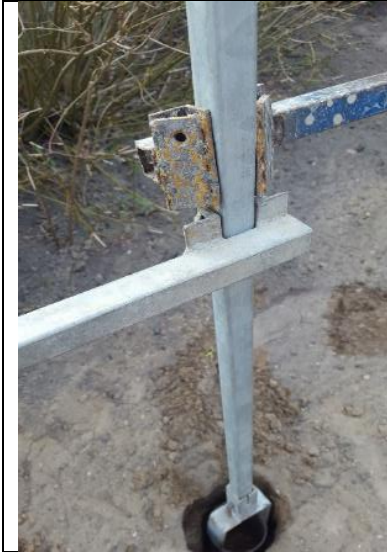
Photo 2. Choose the diameter of the auger. In this case a 4 inch auger for a 4 inch casing.
