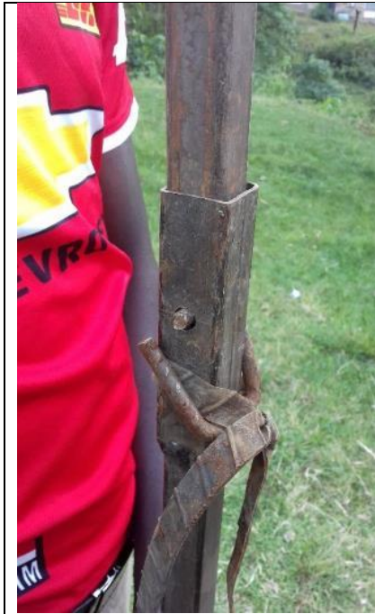
Photo 6. Connecting a new pipe with Fast fix pin. Secure the pin with a rubber strip
