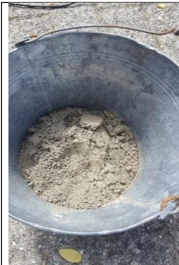
Photo 25. Prepare concrete (1 part cement, 2 parts sand) and very little water, so concrete is like clay
