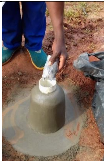
Photo 26. Put concrete in a small plastic bag and make a knot. Shape it like a cigar and drop in casing.
