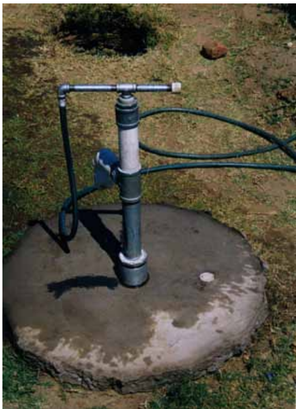
Top photo: EMAS pump installed at a family farm in Nicaragua.
