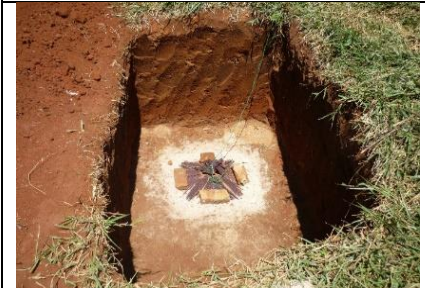
Tube recharge. A technology to store 100-500 cubic meters of rainwater per year or more in the ground. Material 10$
