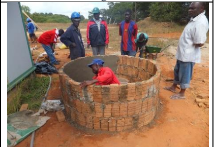
Wire brick tank. Water storage tanks using wire and bricks of cement blocks. Volumes of 1 to 50 cubic meters. Over 400 installed
