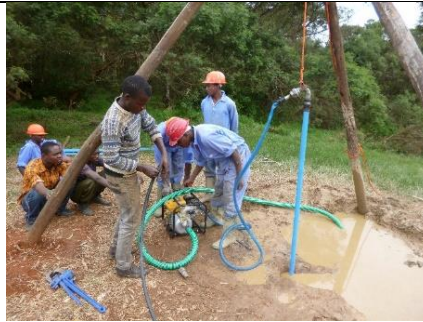
SHIPO drill with jetting. The SHIPO drill combined with a standard engine pump for jetting. Tungsten drill bits added for hard soils
