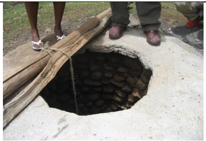
Well ring reducer. A system to reduce the top of the well in order to install a well cover. A well cover and pump will be installed later
