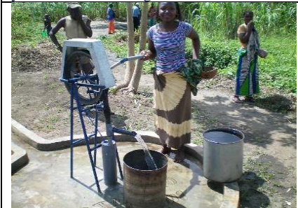
Open well after upgrade. This well is upgraded to an improved water source using a well cover and Rope pump
