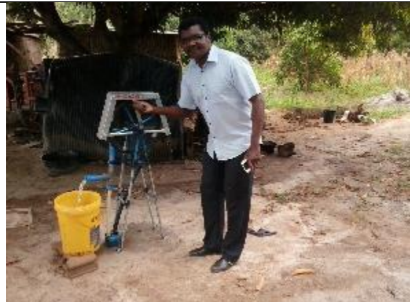
In this case in Maputo the 6 meters deep Tube was made in 1 day and a Rope pump is installed on a prefabricated slab
