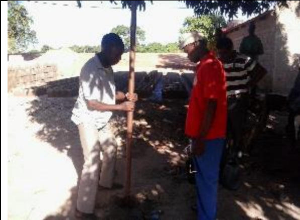
Making a Tube well with the Mzuzu drill Method, The first 3 to 7 meters is made with a Soil punch
