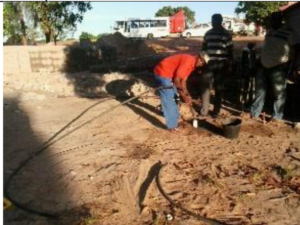
Making a Tube well with the Mzuzu drill. After a first hole with the Soil punch the casing is placed and lowered by using a Tube bailer which pumps out sand inside the casing.
